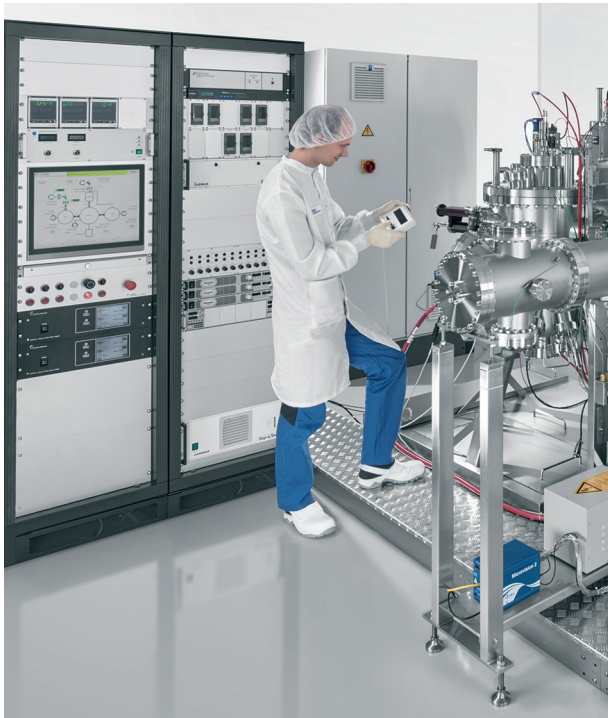
System control rack
